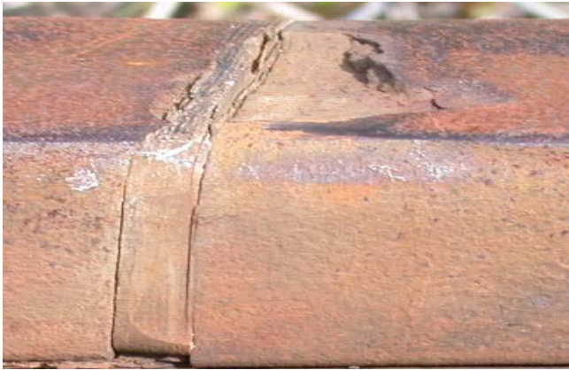
Fig. 8 A Typical IRJ Failure (Chipping Out)
