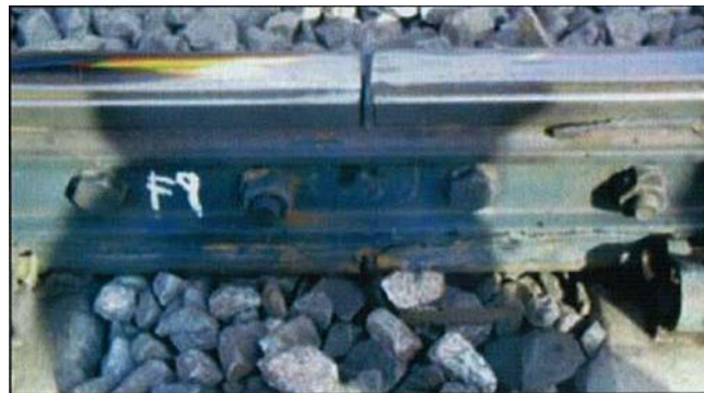
Fig. 5 End Post Crushed in IRJ Due to Pull-Apart
