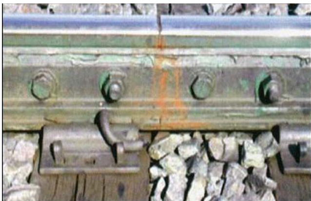
Fig. 4 Failed Glued Bond in IRJ
