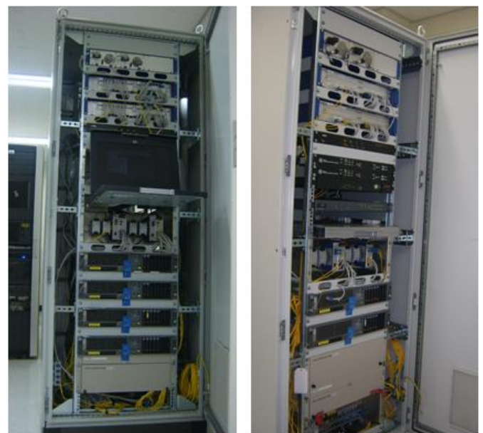
Fig. 4. SCADA Servers and Industrial LAN Switches in LCC
