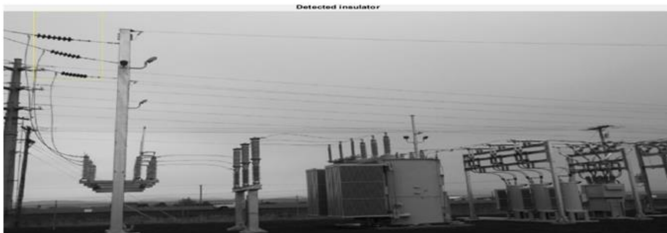
Fig. 13 Location of insulator in a cluttered scene
